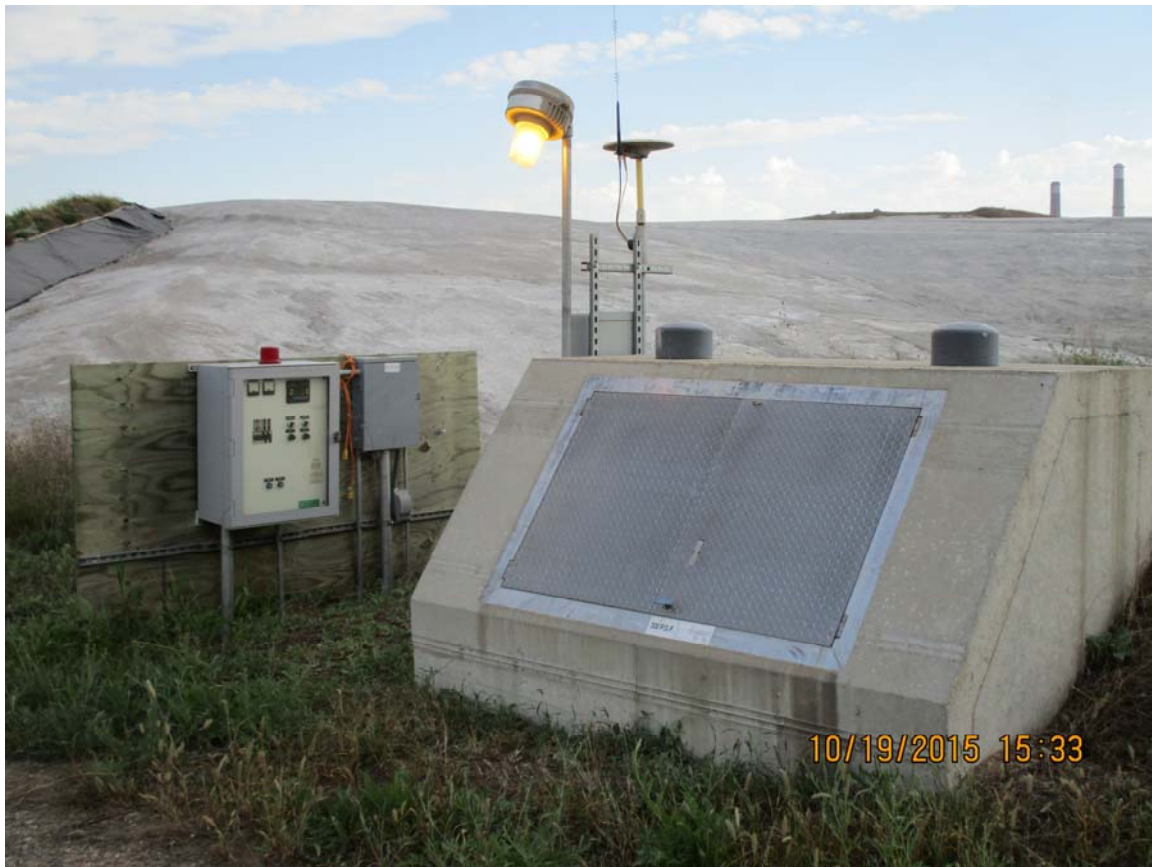
Photo 9 Left: Cell 2C Pump Controls. Right: Cell 2C Riser Pipe Access Panel 10/19/2015
