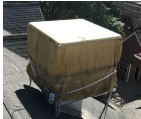
Example Evaporative Cooler with Cover
