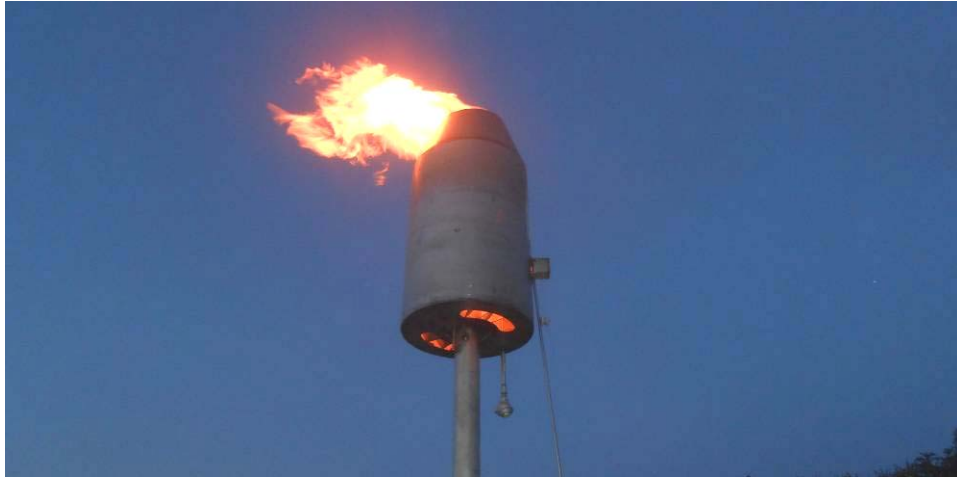
Photo 11: Gas flaring off the digester when the generator is not in use.
