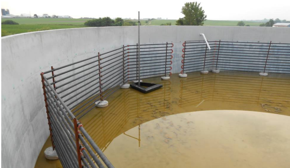
Photo 9: Hot water from cooling the engine flows through these tubes to heat the manure
