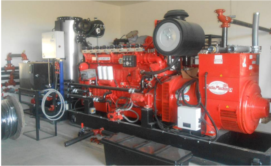
Photo 13: The engine that will produce the electricity
