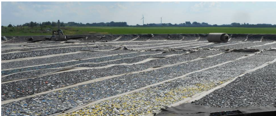
Photo 10: The layer of insulation between the layers of plastic forming the digester cover
