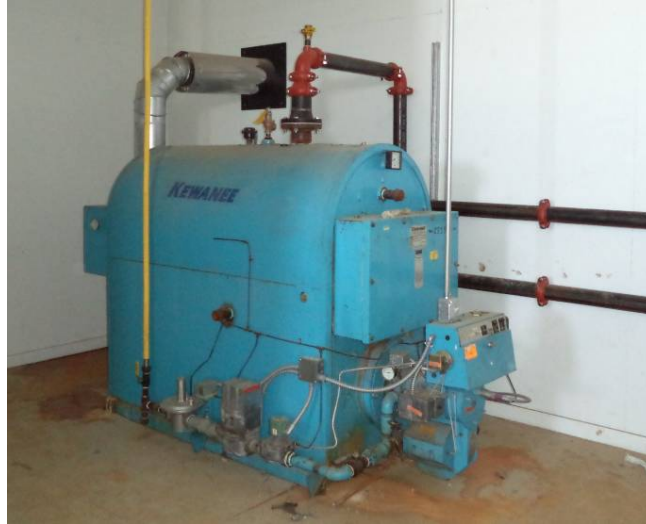
Photo 14: This boiler was purchased and retrofitted to burn the gas collected in the digester. It was used to bring the digester up to temperature initially and will be available for back up heat if needed.
