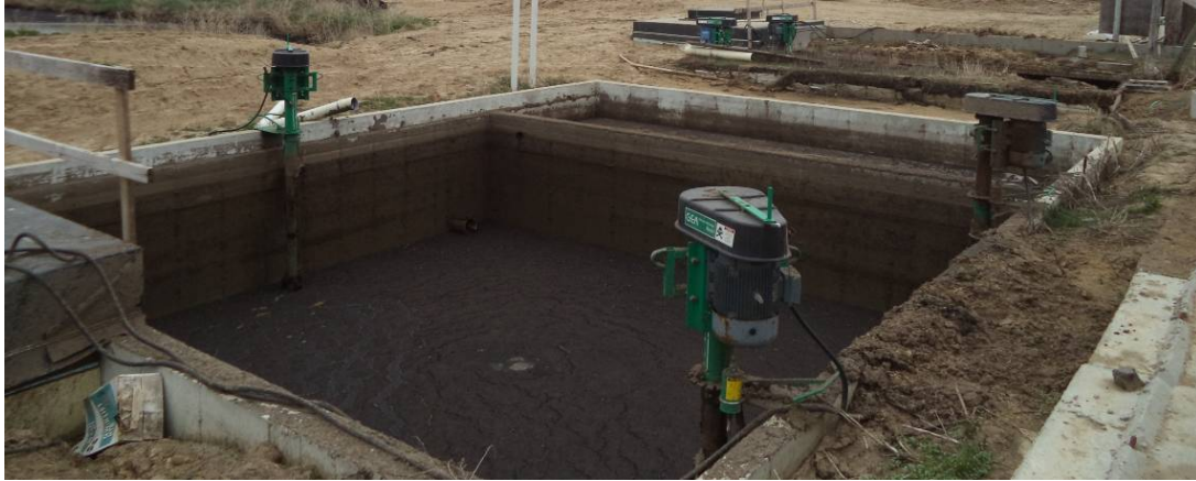
Photo 7: The digested slurry flows into a pit from which it is pumped to the separator building.
