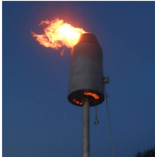
Photo 13: A flare has been constructed a safe distance away to burn the gas if the engine is being serviced or otherwise off line.
