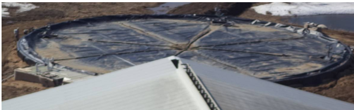
Photo 12: The digester vessel is a round concrete structure covered with a specially designed, sealed, floating insulated cover to capture the gas.
