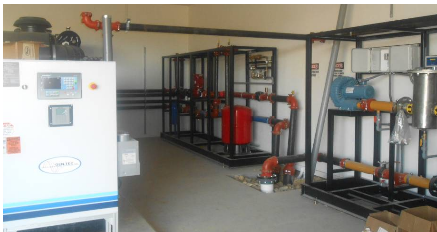
Photo 8: The skid on the right side of the photo brings the gas into the engine room. The one on the left circulates the hot water.
