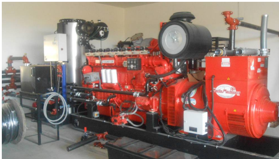
Photo 15: A Guascor engine is used to generate electricity from the methane.
