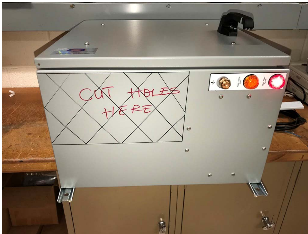
Image 2. The area on the outside of the cabinet where the Customer can drill holes to attach conduit terminations for power and communication.
