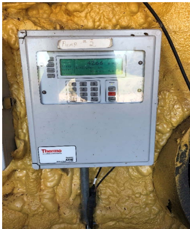
Photo 10 Display screen on properly functioning Pump No. 2. 10/24/2019
