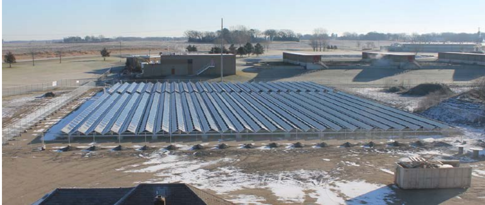
Photo 2: 400 kW DC array on a closed municipal landfill in Hutchinson
