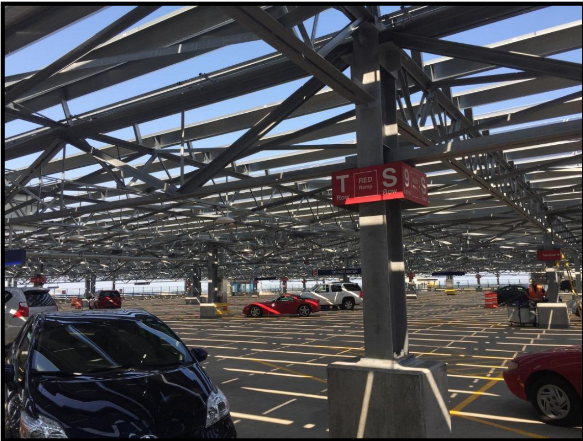
Covered parking is a related benefit of the solar systems on the Red and Blue parking ramps. The superstructure and panels provide relief from harsh winter and summer weather.
