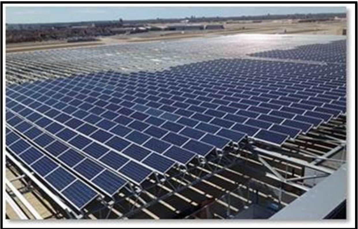
Panels were oriented to capture optimum solar radiation while complying with FAA rules that eliminate or minimize glare for approaching aircraft.
