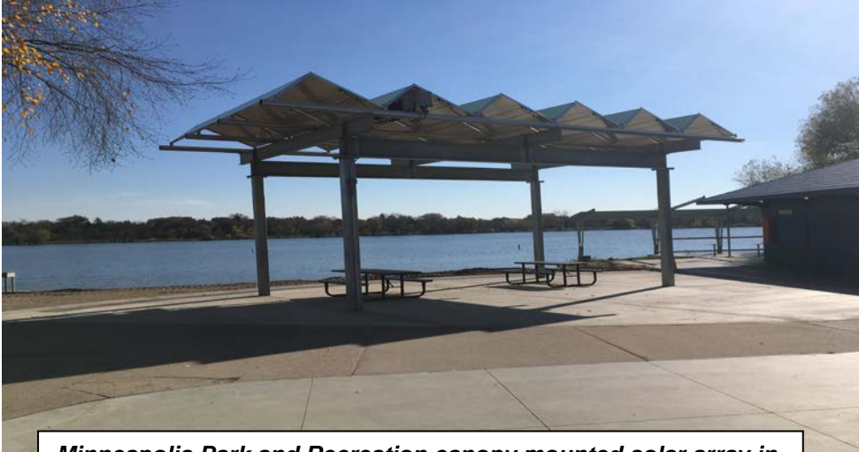
Minneapolis Park and Recreation canopy mounted solar array in Minneapolis, Minnesota, A RDF-funded project
