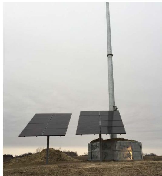
Figure 3. North Site with 4kW Solar Array
