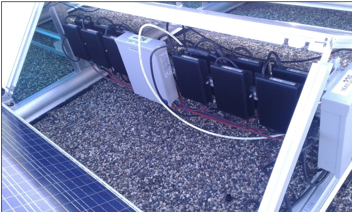
Inverter Bus at 2550 University Avenue
