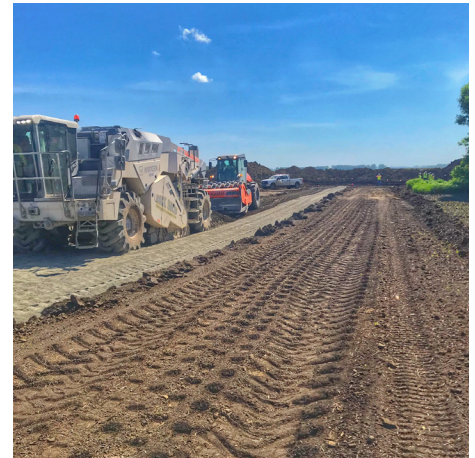
Access road grading and gravel placement is the first step of construction.
