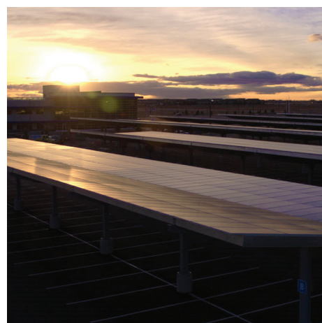
The 1.3 MW ac carport solar installation started producing power in March 2017.
