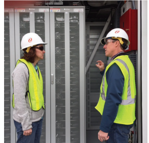
Xcel Energy employees look at a bank of Younicos Y.Cubes that compose the Panasonic battery.
